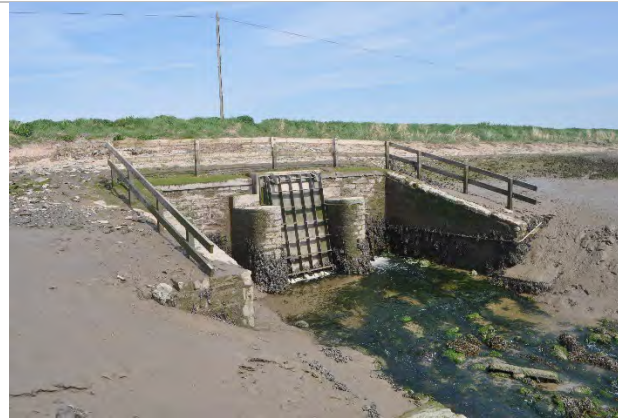
Plate 3.12 Downstream side of the Great Sluice. Water from Braunton Marsh discharges to Horsey Island.
