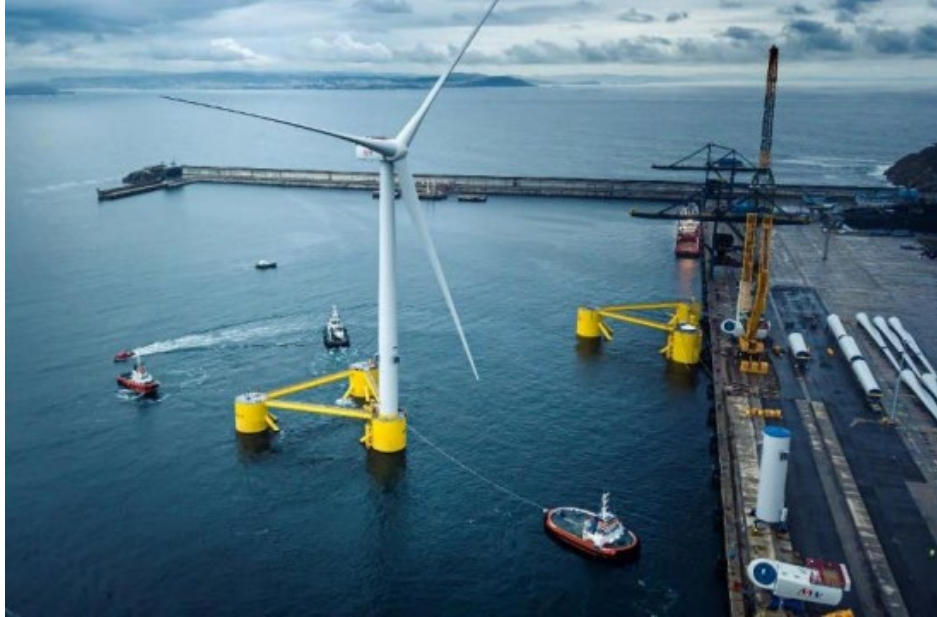
Plate 5.13 Example of WTG assembly onto a semi-submersible platform at quay side (Source: Photo courtesy of Principle Power)
